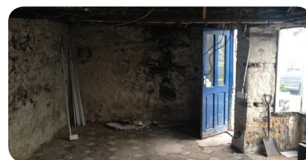
The gutted shop interior.
